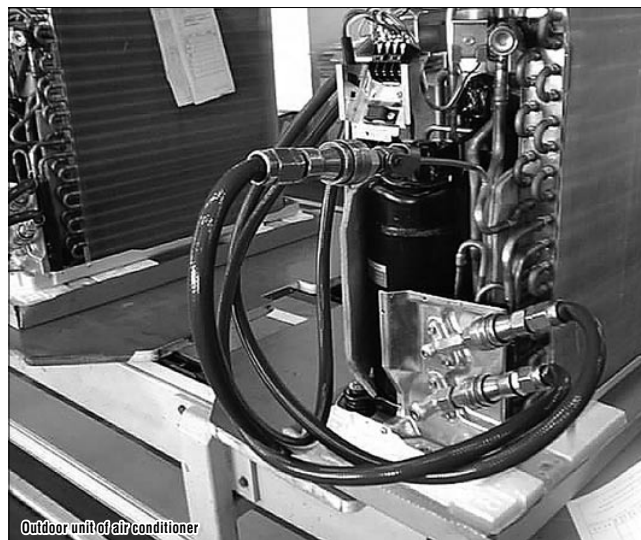
Outdoor unit of air conditioner
